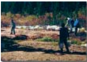
Top: Tailings-tainted runoff makes its way toward the St. Mary's/Alice subdivision prior to the project. Middle: A crew prepares the French drain. Bottom: Volunteers spread ground limestone on tailings deposits in Little Creek.
