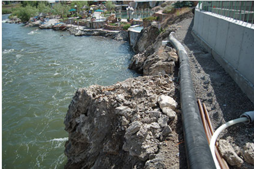
After crossing the pedestrian bridge, the black pipe continues along the bank of the San Juan toward the Springs Resort bathing pools. A new retaining wall, seen to the right in this photo, is part of an expansion project that will add five additional bathing pools to the resort's existing 18.
